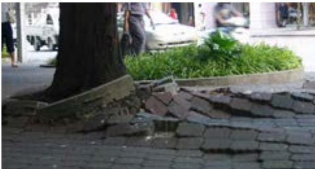
Improper maintenance or tree selection creates hazards.
