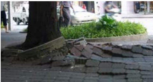
Improper maintenance or tree selection creates hazards.
